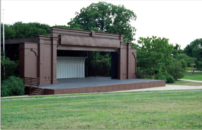
The Sylvan Theater is not oriented to take full advantage of seating on the hillside south of the Washington Monument. Infrastructure is outdated for performances.
